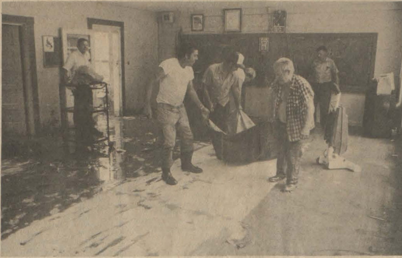
Workmen remove damaged carpeting from a classroom building at McDowell High School following Thursday night's flash flood.
