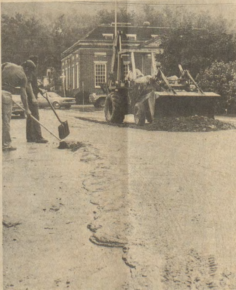
A CITY WORK CREW shovelled and hosed tons of mud from Court Street here Monday, after heavy rain Sunday night had washed it from the hills above the city. After clogging the drain at the intersection of Court Street and Lake Drive, mud and water backed up, entering several business premises nearby. A construction site for a new house at the crest of Court Street was cited as the source of much of the mud. City Manager Jack Clark Hyden said that the city should consider requiring a retaining wall before issuing a building permit in such cases.
