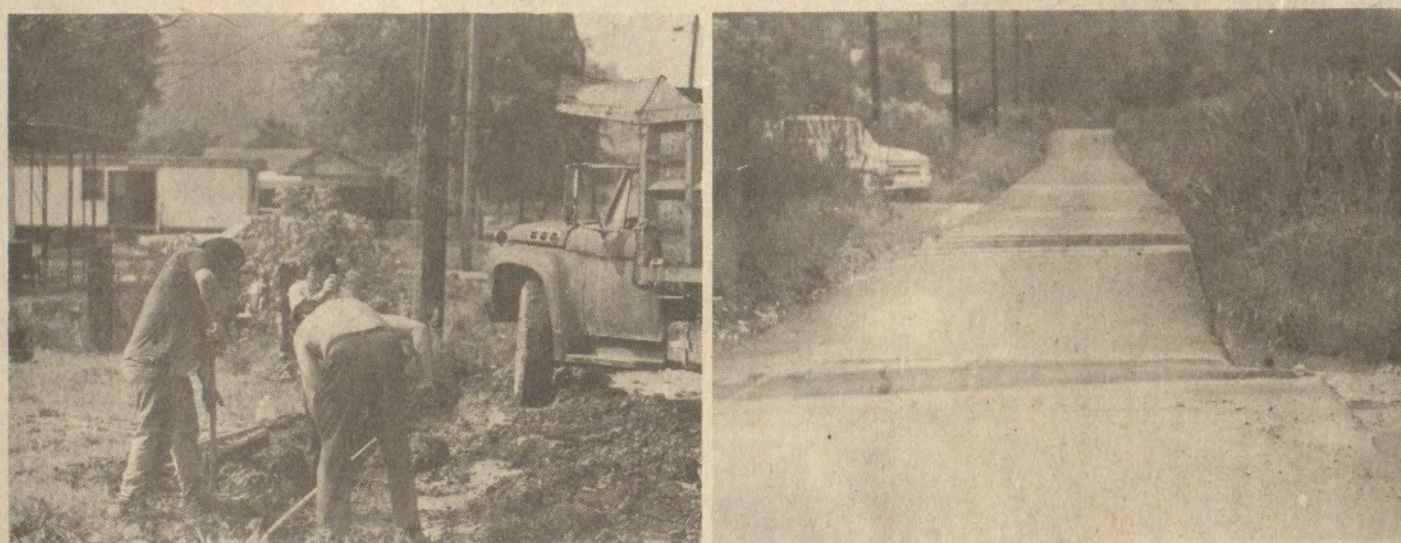
In photo at left volunteer workers dig a ditch along a Dwale roadway in an effort to remedy drainage problems which plague the community's lowest end. Problem is typified by photo at right.
