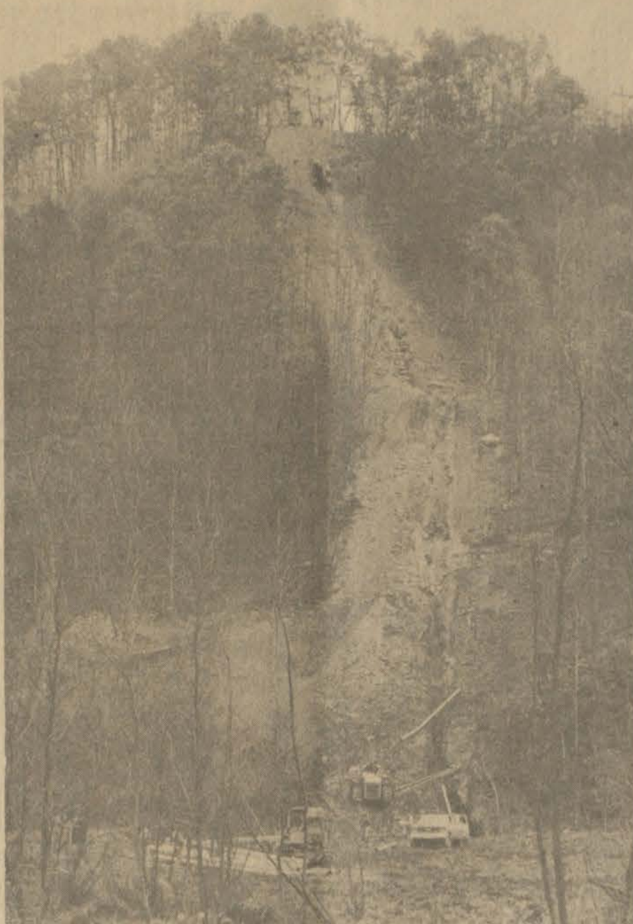
NEW KY 80 CONSTRUCTION will mean the displacement of miles of pipeline along the route and many lines have already been moved or are in the process of being moved. The relocation work pictured above involves line along Rock Fork Creek near the Floyd-Knott county line.
