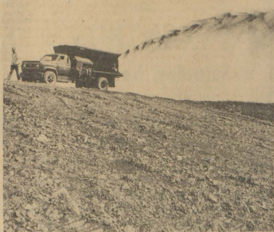
Bark Spreader works its way across an experimental plot on the Ken Lick Coal Company strip-mine in Breathitt county.
