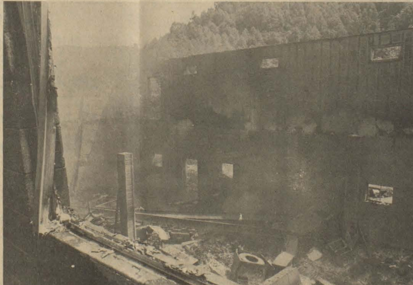
Fire early Monday morning, destroyed the block building (formerly the Martin Youth Center) which housed the Ornamental Iron Works Co., a firm which only recently moved into the structure on Route 80 near Martin. The blaze, apparently originating in ceiling wiring, resulted in more than $100,000 damage including the loss of seven welding machines and a large quantity of stock.
