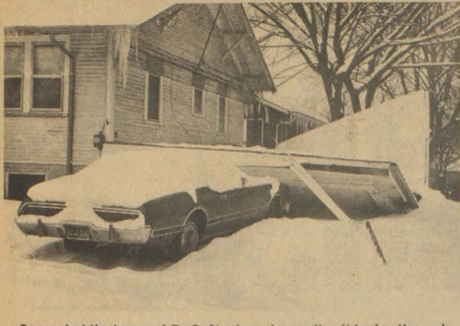
Carport at the home of D. C. Stephens here after it had collapsed beneath the heavy load of snow.
