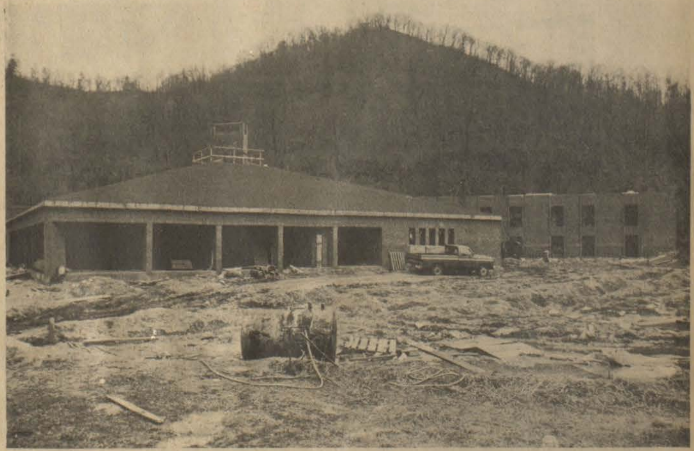
Although completion of the new $1.8 million Riverview Manor is not expected before early fall, the 116-bed extended care facility was under roof when this picture was made this week and some inside finishing work had begun. The two-story structure, which is being built on a two-acre tract adjacent to Briarwood Addition here, will offer 56 skilled and 60 intermediate care nursing beds. Owners of the facility are P. & P. Investment, Inc., of Prestonsburg, and contractors on the project are Gold Key Builders, of Dayton, Ohio.
