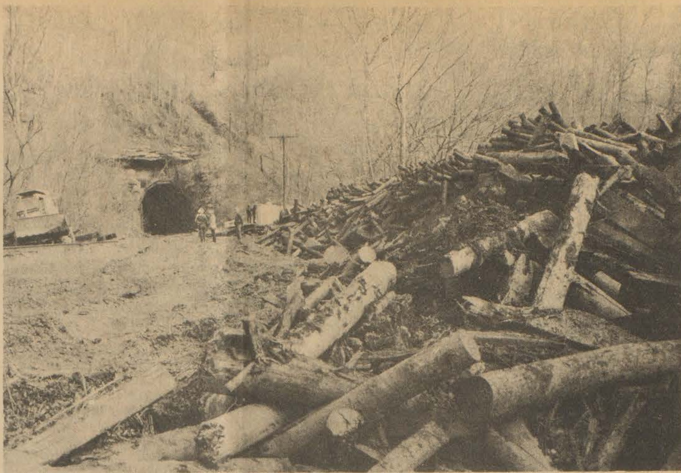
Debris removed from Stephens Branch tunnel by railway employees during five-day effort to clear tracks for traffic after wreck.
