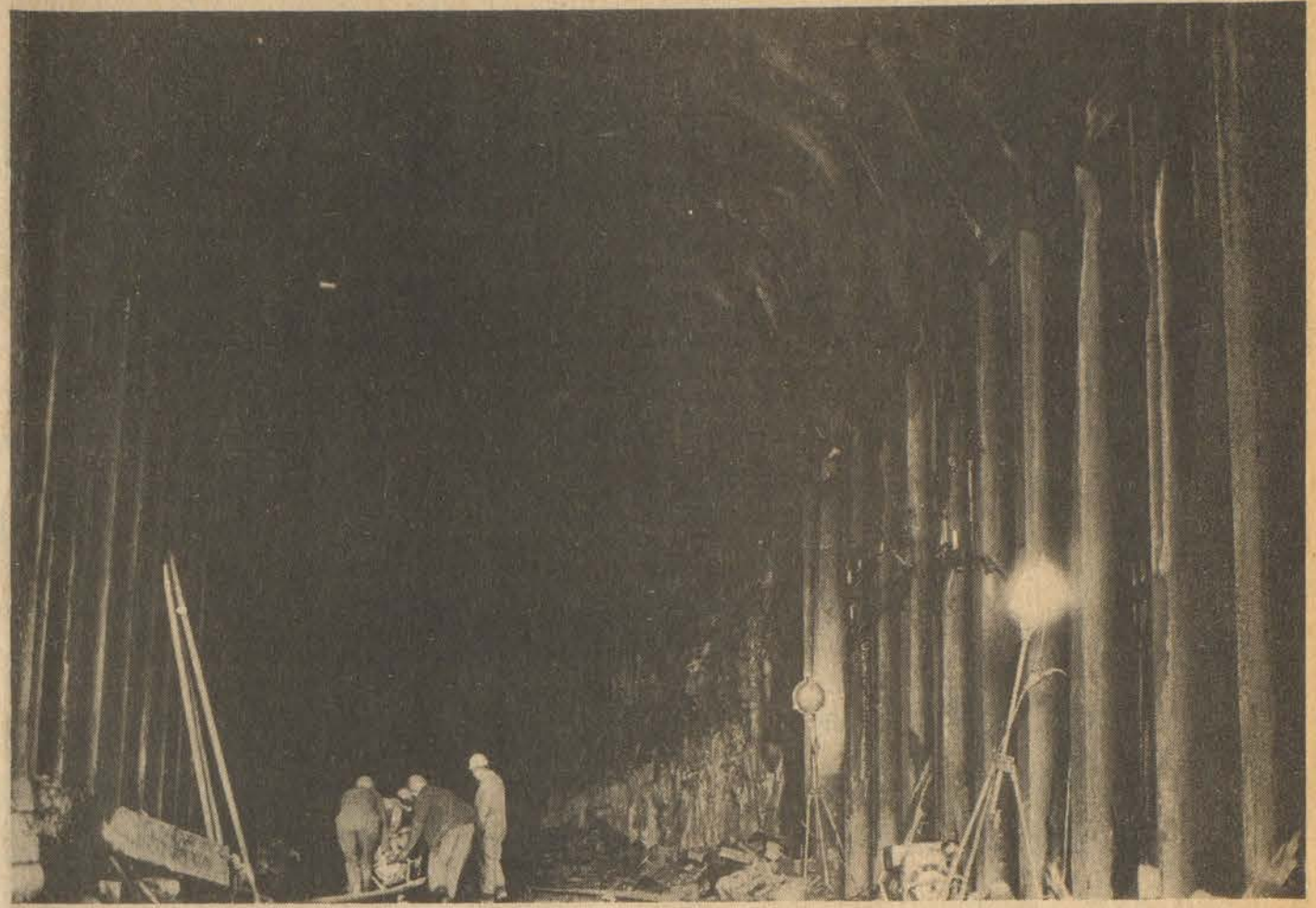
Interior of tunnel shows where supporting timbers were torn away by wreck.
