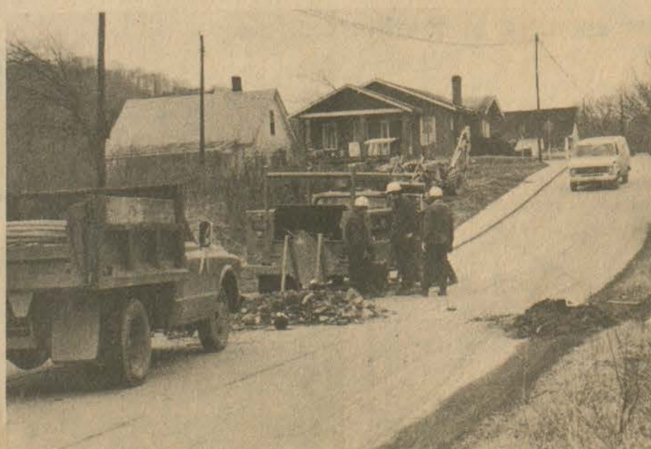
Water and Gas Commission crew at work on Highland Avenue near grade school.
