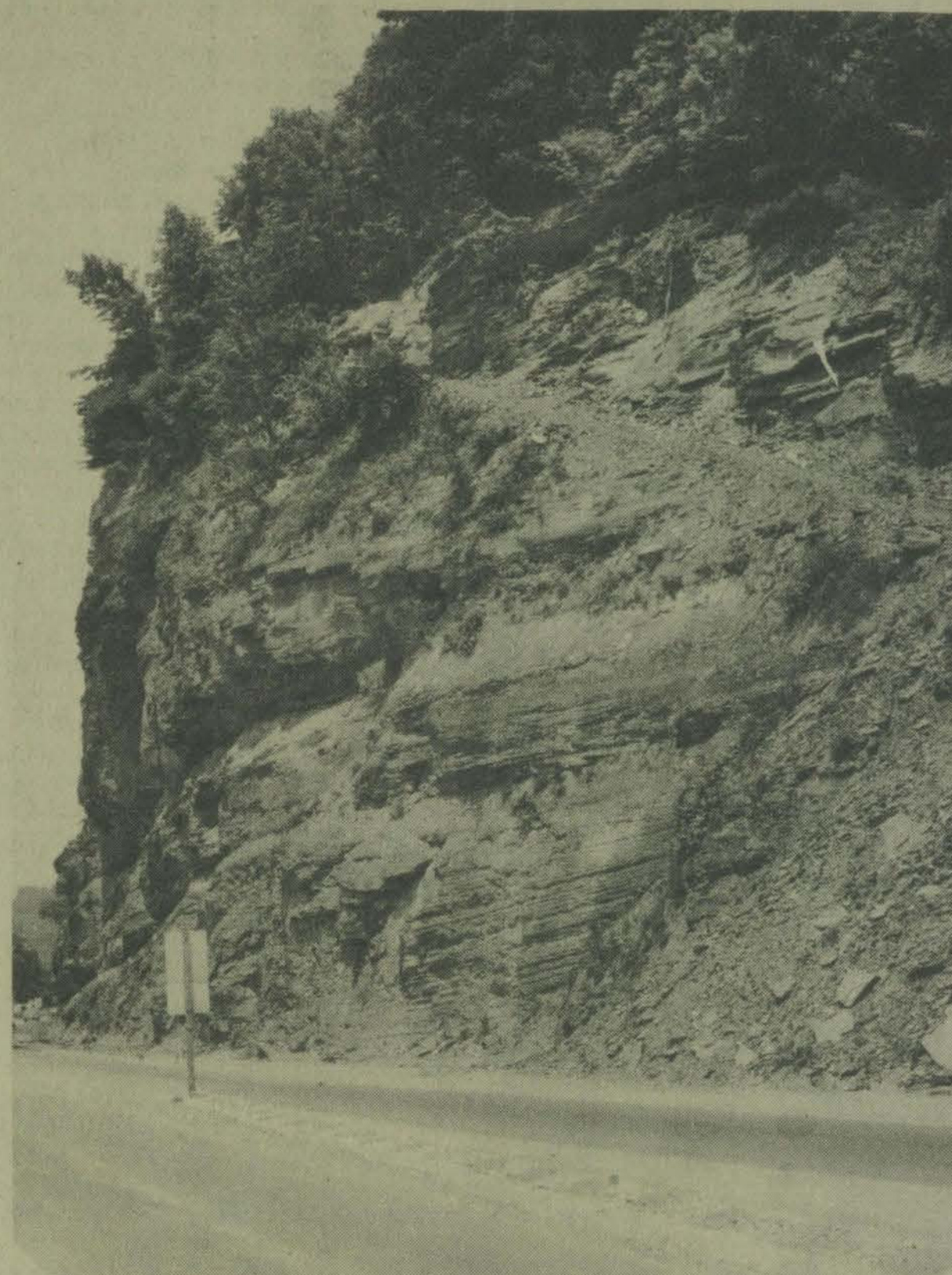
This road cut on U. S. 23 North, in Prestonsburg, continues to hold area motorists in suspense as they pass under the overhanging sandstone boulders which rest on crumbling layers of shale. The site of numerous rockfalls and resulting accidents, work which was begun last winter to shave the cliff face away from the highway was abandoned and no further efforts have been made to finish the much needed project.
