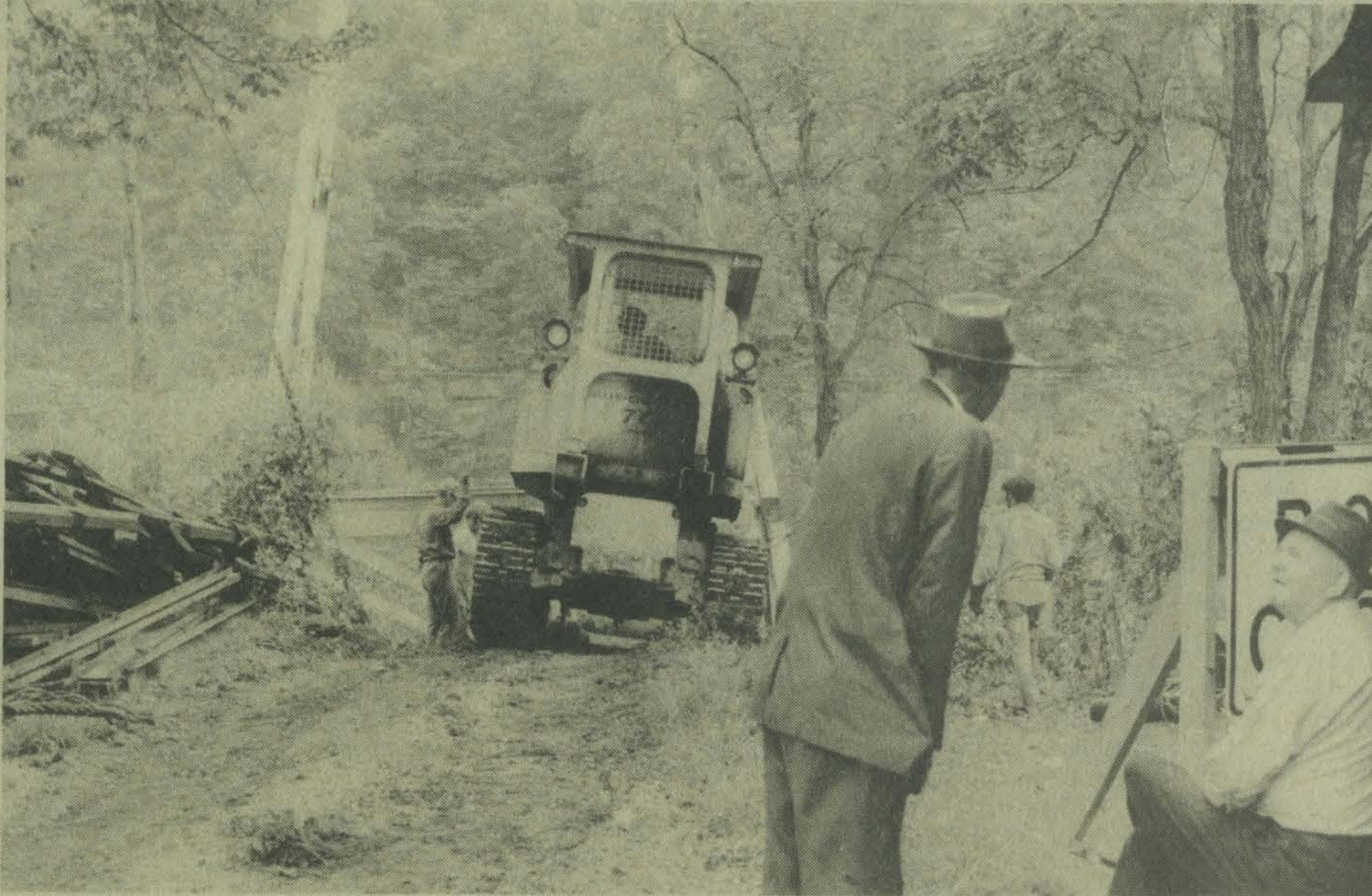
They tore down the old bridge at Emma last week, soon after the new $439,899 span across the Big Sandy there was opened to traffic. In photo residents of Emma are interested spectators as machinery is being used to haul down the superstructure of the 47-year-old landmark. Some of those who live at Emma said they would have preferred to see the old bridge stand and be used for pedestrian traffic, but one pointed to old bolts from the bridge which were almost rusted in two. "It would have fallen before long, anyway, and somebody might have been killed," he remarked.
