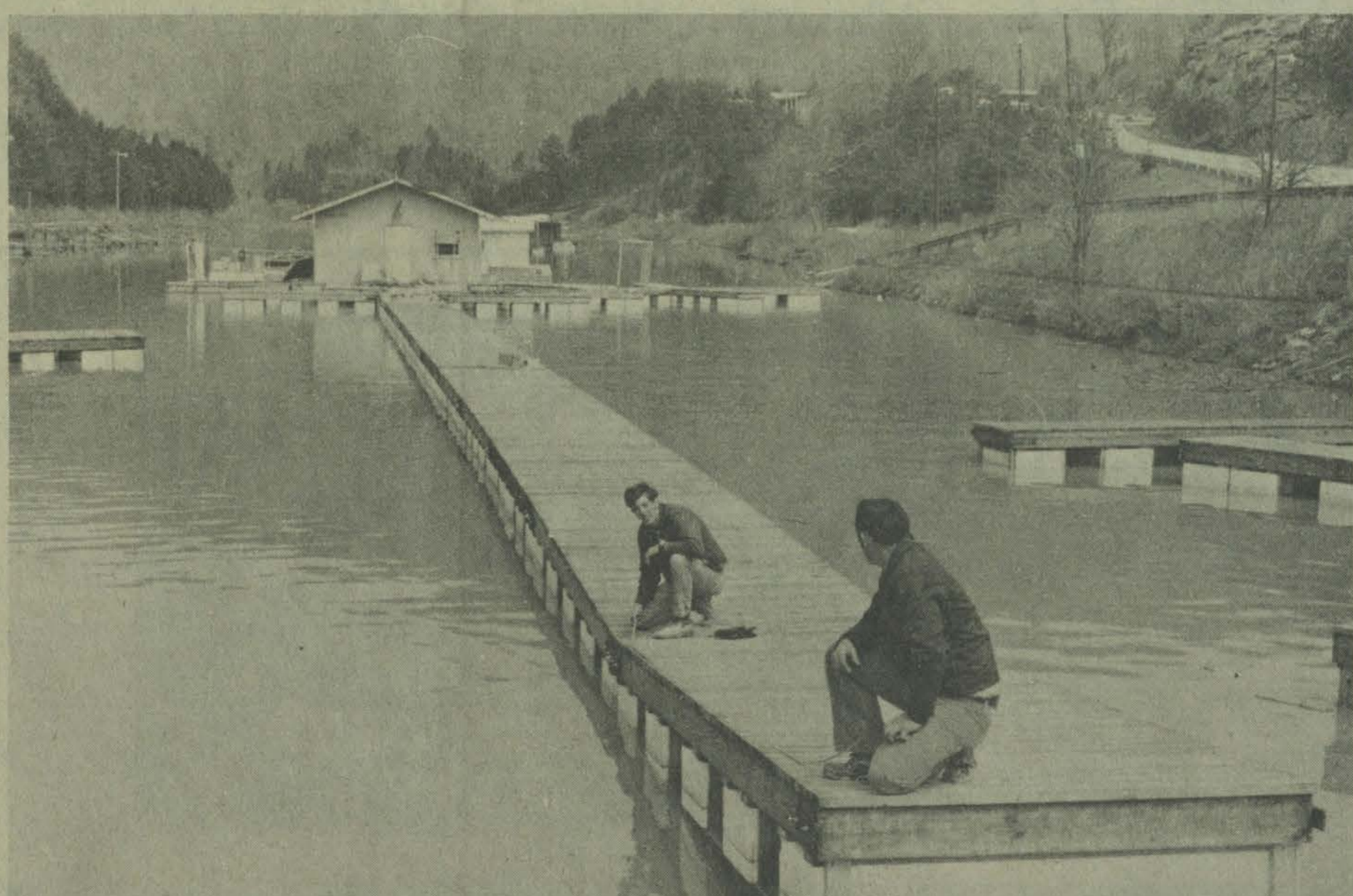
The first stage of improvements at Jenny Wiley boat dock is well under way with the construction and installation of an entirely new section. A total of $2.5 million has been earmarked for improvements at the dock and other work within Jenny Wiley State Park.
