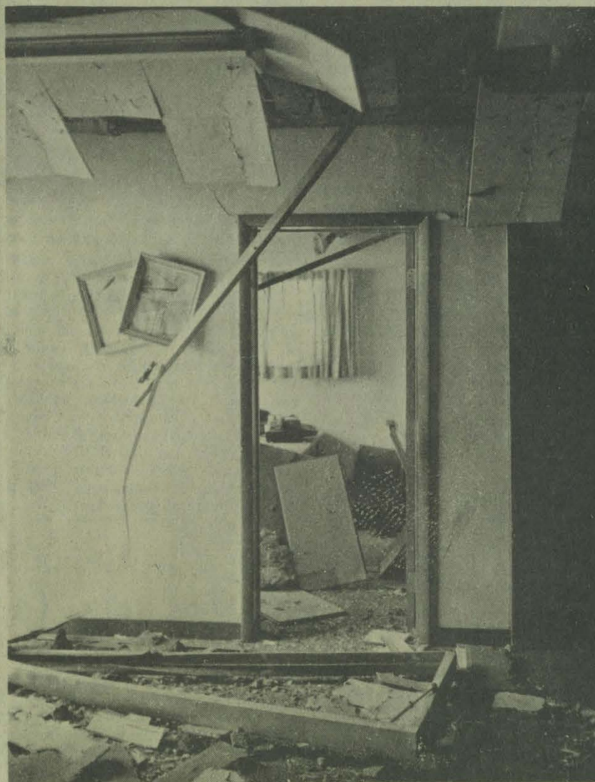
Interior of company office. Fragments of front door on floor and hanging from ceiling.
