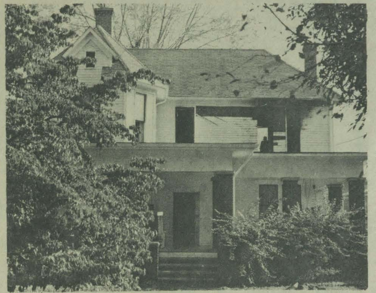
The Sally G. Clark home on Arnold Avenue bears evidences of fire which damaged the roof and second floor last Friday morning. Water and smoke damage to interior of the residence and its contents was heavy.
