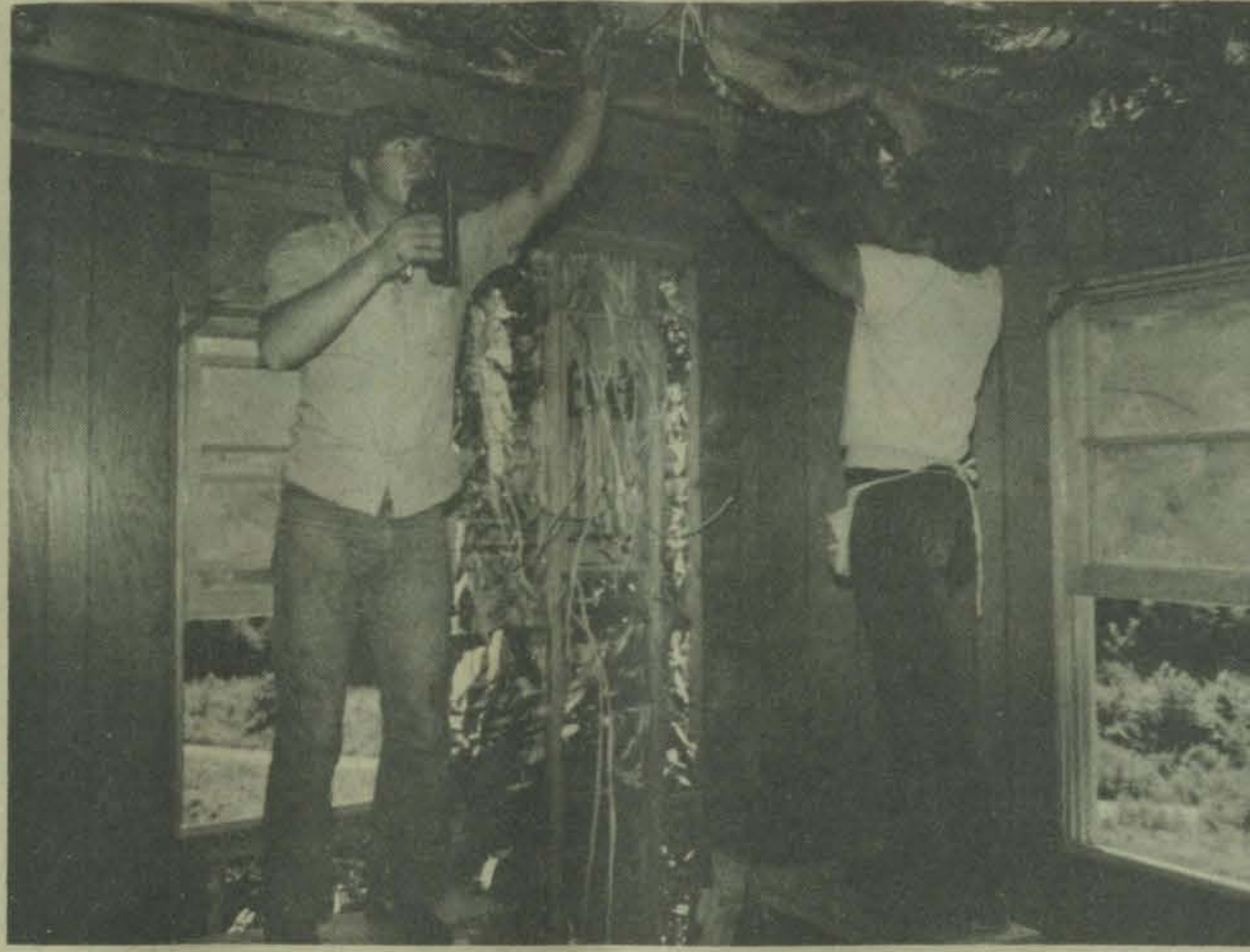
Two Hueysville trainees—Vondel Shepherd (left) and Clarence Slone—prepare to install ceiling tiling in caretaker's home.
