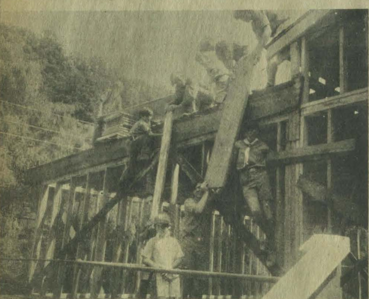
Scouts (top photo) at work on David Community center. Bottom photo shows second story of building partially completed.
