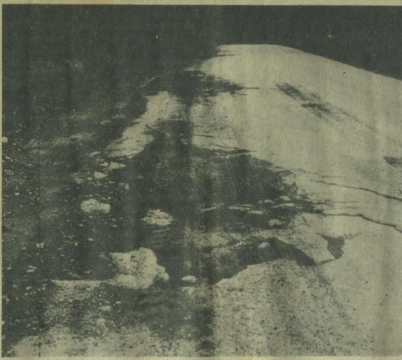
Photo shows some of damage suffered by Dewey Lake road, apparently the result of heavy coal truck traffic.
