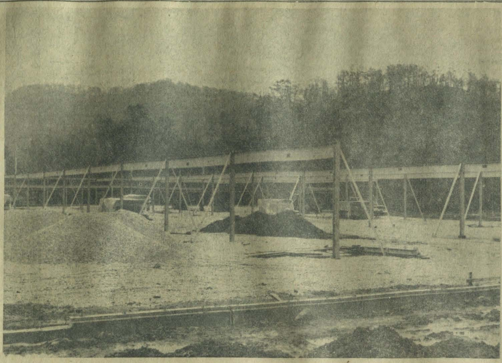
SHOE FACTORY GOING UP. Photo shows first steel erected in a section of the U. S. Shoe Company plant, near Lancer. The plant is scheduled to begin operation next spring.
