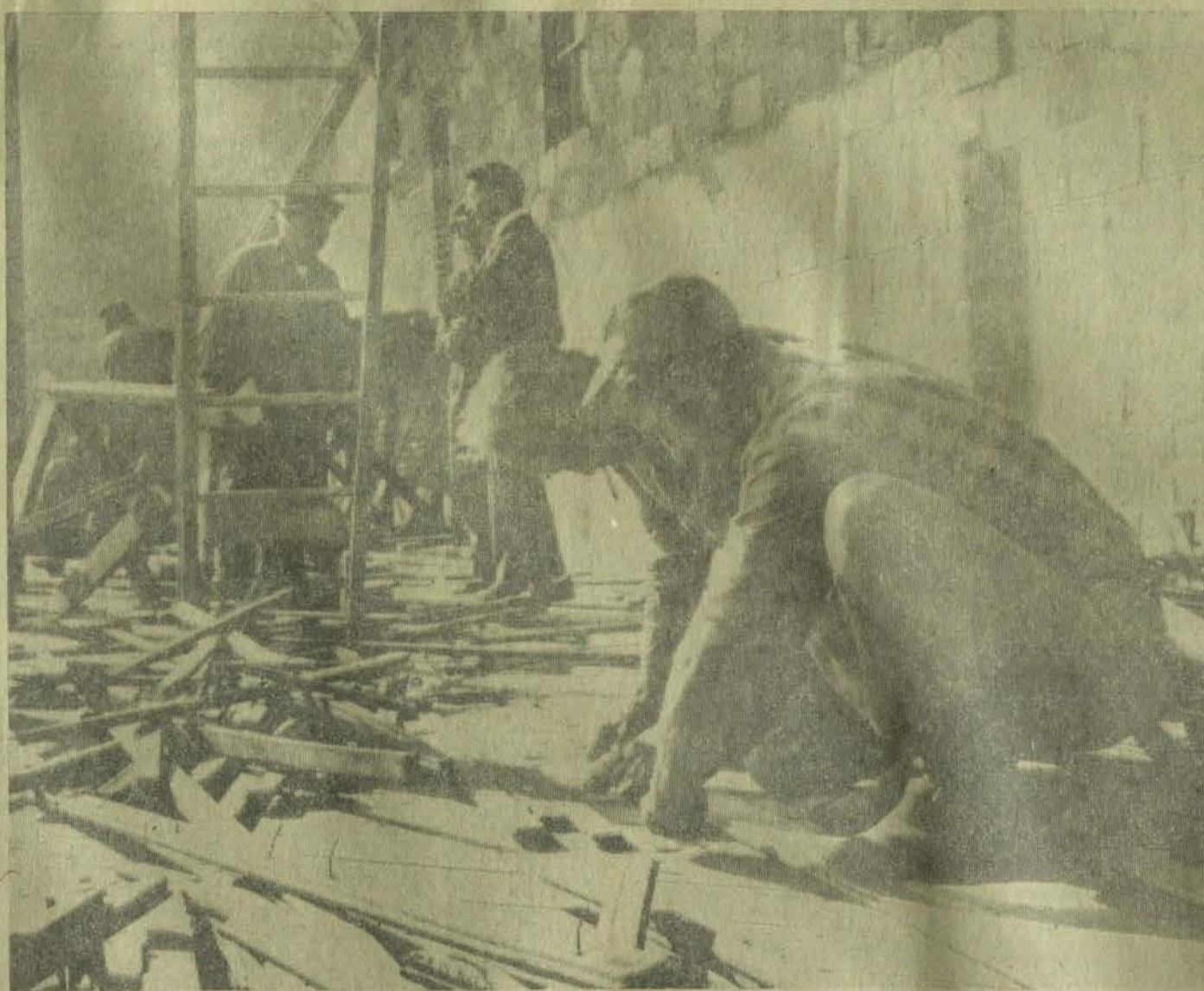
Charlie Prater and Clinton Fraley, participants in the Work Experience and Training Program for unemployed parents of Floyd county, are shown laying flooring on one of the buildings in Archer Park, West Prestonsburg. Nello Francis, county project supervisor, is seen in right background.
