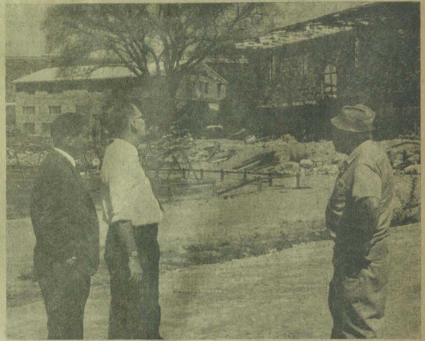
County Project Supervisor Nello J. Francis, Dr. George P. Archer, mayor, and City Manager Curtis Clark, of Prestonsburg, view work done on Archer Park, West Prestonsburg. The planning and drive for the project have come from Dr. Archer and Clark, with the cooperation of County Judge Henry Stumbo. The labor has come from Work Experience and Training Fathers, largely, and is one of the most dramatic examples of such work in the 19-county project.
