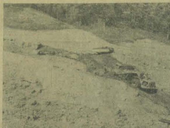
Building the Winchester-to-Campton section of the Mountain Parkway was no easy job; many said it couldn't be done. More equipment, machinery and manpower were concentrated on its construction than on any road project in state history. Curves are broad and gentle. No grade is steeper than seven per cent. Giant cuts—up to 260 feet in depth—permit the easy slopes.
