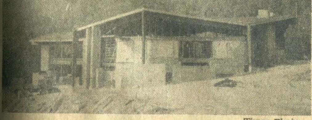
JENNY WILEY LODGE . . . Akers & Akers, contractors on the Jenny Wiley park lodge, will complete the structure by July 15, it is said. The lodge and adjacent 35 living units will cost approximately $800,000.
