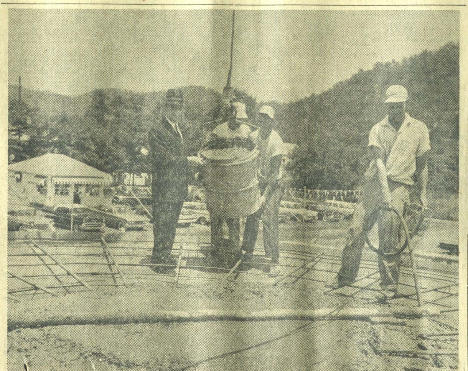
BANK BUILDING UNDER CONSTRUCTION . . . Construction of the Allen branch building of the Bank Josephine, started in June, is expected to be completed by Nov. 1, according to H. D. Fitzpatrick Jr., vice-president of the parent bank. The Allen bank will have drive-in as well as conventional banking facilities. Mr. Fitzpatrick, left, is shown here as the concrete base of the building was being poured.
