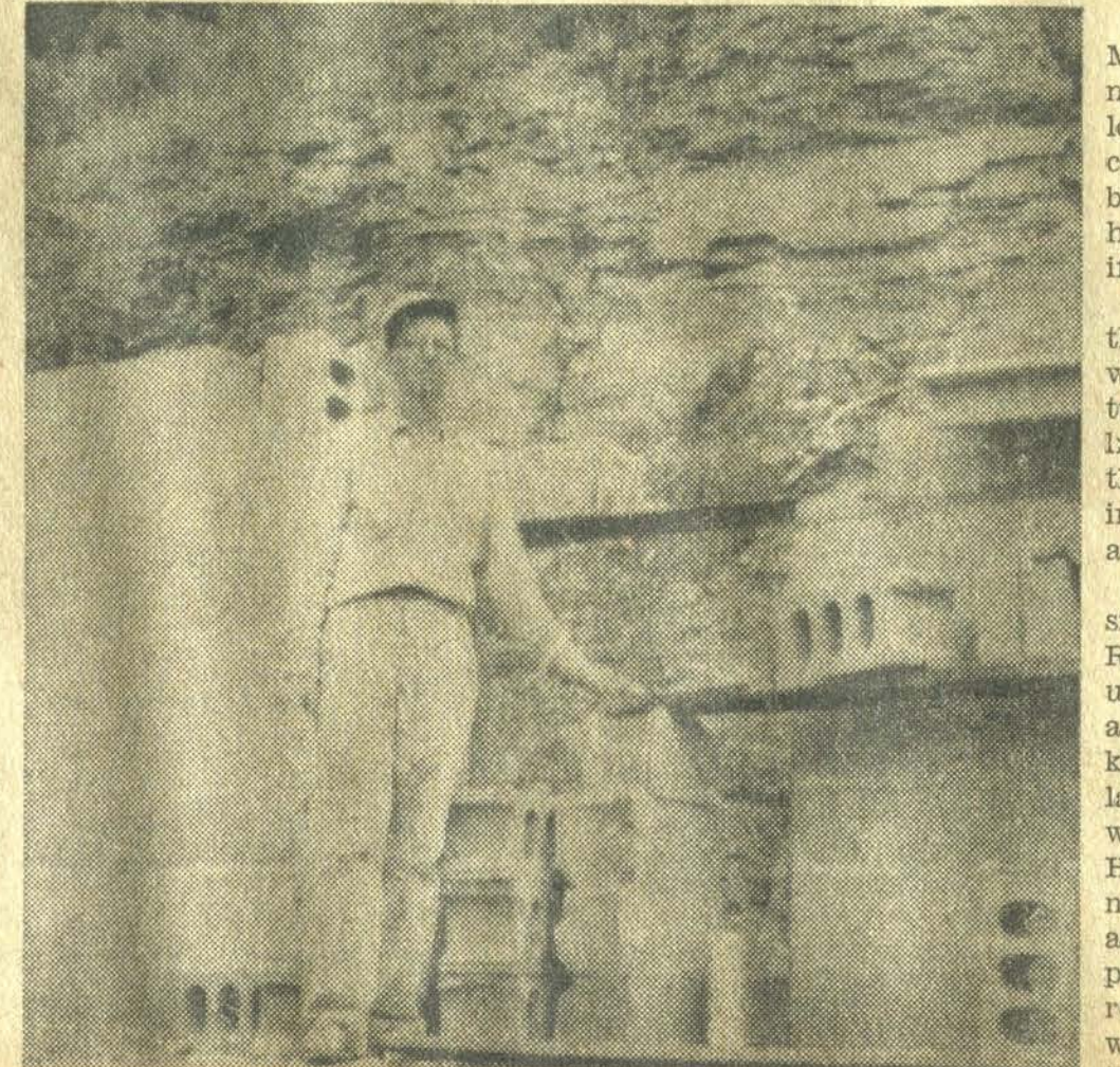
Rev. Robert Martin, 48, former pastor of Dock Community Church and Grace Chapel in this county, repairs the hole wrought by a giant boulder when it plunged through the wall of the church he is building at Martin.
