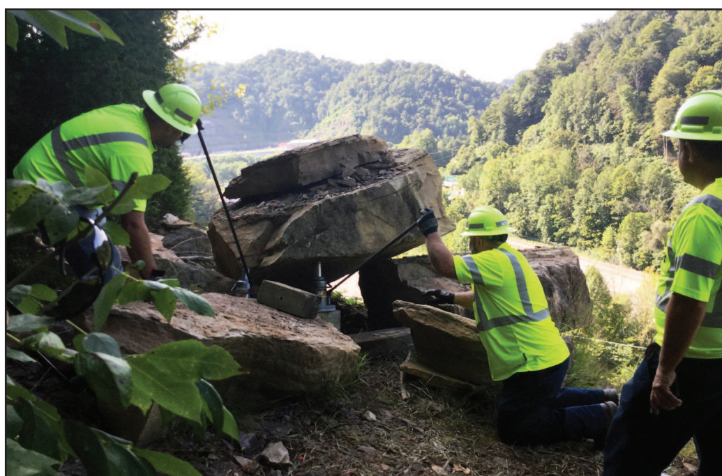
Submitted photo Workers from the Highway District 12's Minnie Maintenance department saved more than $100,000, the department reports, by removing these boulders on the hill on Rt. 80.
