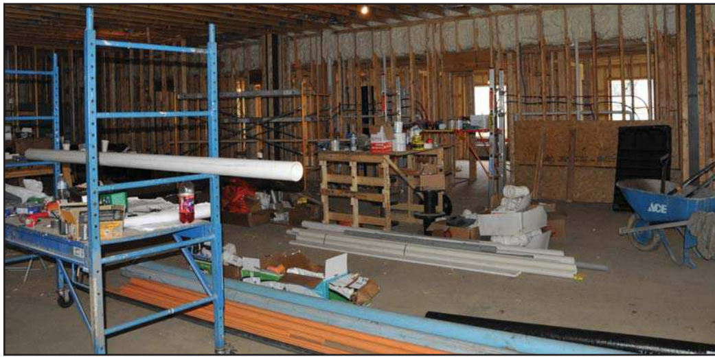
Floyd Chronicle and Times photo by Mary Meadows Interior work is still underway at the Walter K. Bowling Homeless Shelter, which was expected to open last year. The opening has been delayed because of the lack of funding, VFW officials say.
