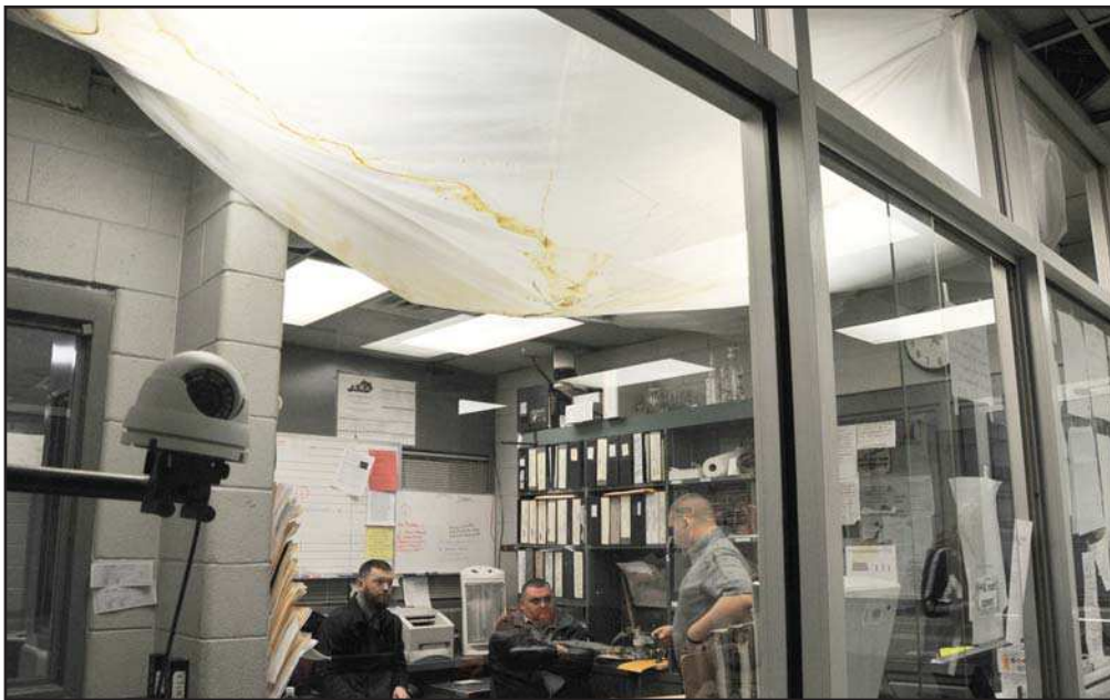
Floyd Chronicle and Times photo by Mary Meadows Floyd County Detention Center employees have been battling a leaky roof on the facility for years, a problem Judge-Executive Ben Hale blamed on the lack of maintenance in prior administrations. Jailer Stuart "Bear" Halbert said the problem is now "uncontrollable." Officials are planning a jail roof replacement this year.
