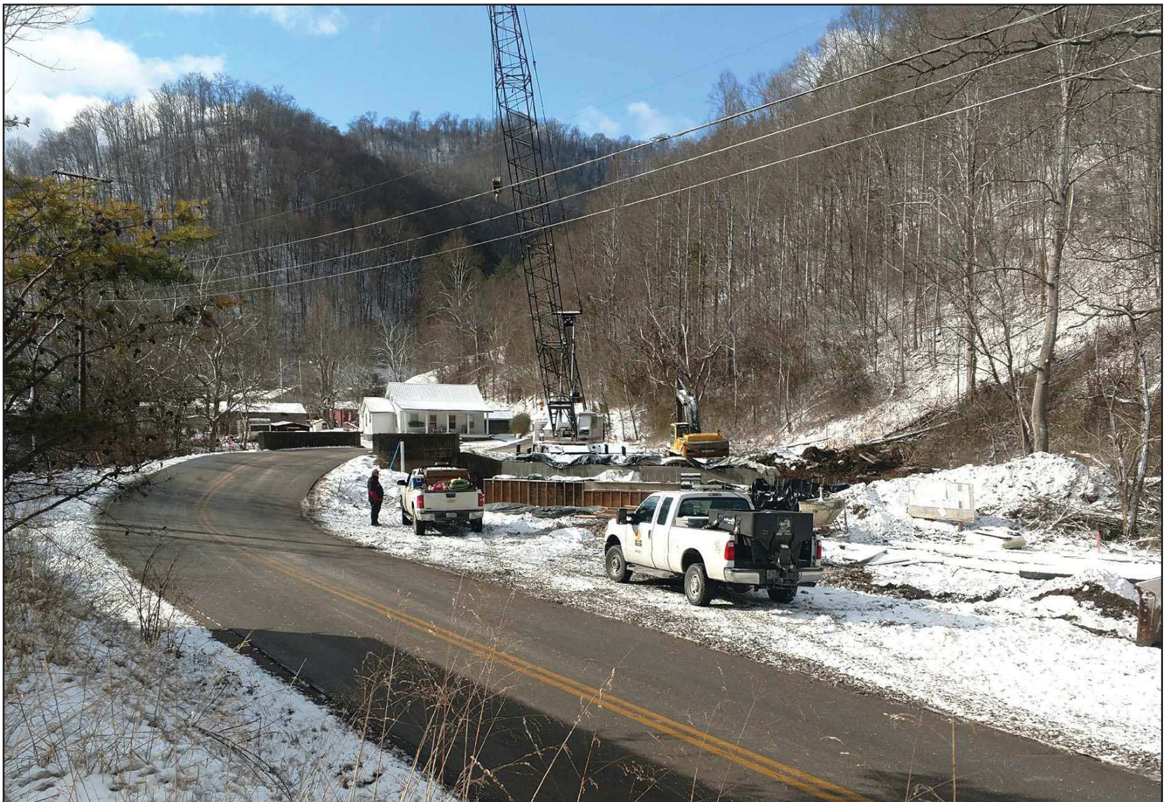
Submitted photo Highway District 12 officials work with bridge contractor Frederick & May of West Liberty on KY 466, building a new bridge on the Left Fork of Beaver Creek at Melvin in Floyd County.
