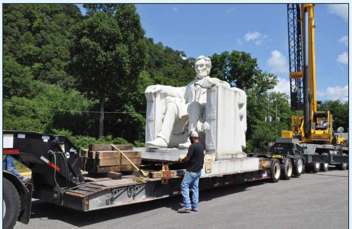
Appalachian Newspapers photo by Aaron K. Nelson On Monday, Modern Contracting of Stanville removed the statue of Abraham Lincoln from its base at the former law complex of Eric C. Conn. Jerry Flannery, who bought the Conn property after it was seized by authorities, said he was happy to see the statue on its way to a nearby business for refurbishing before it is taken to its new home at the Middle Creek National Battlefield.
