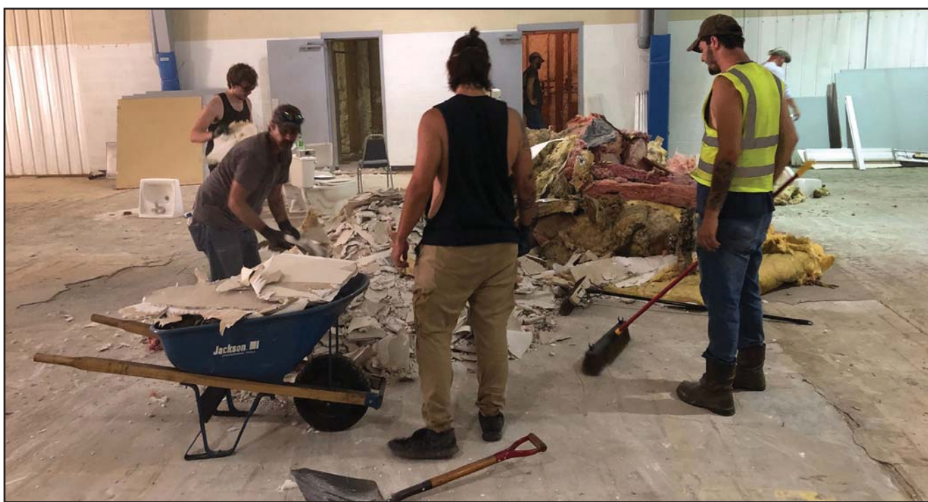
Submitted photo Litter abatement workers, dubbed the "Floyd County Clean Team" by Code Enforcement officer Joe Reynolds spent some time this week clearing out the floor in the former Martin Community Center. The building has been recently painted and flooring still needs to be installed. Judge-Executive Robbie Williams reported that the community center should be ready to open soon.
