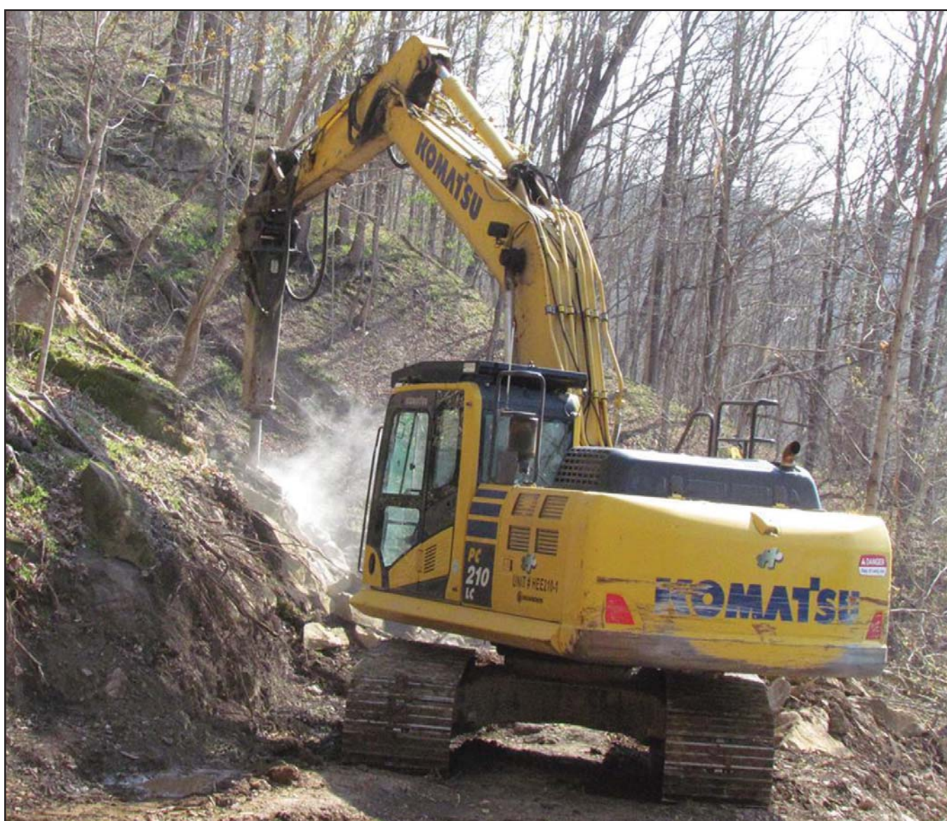
Submitted photo James Young of Jigsaw Enterprises, the state's contractor on the Ivel slide, works the hoe ram attached to an excavator to break up a boulder on the hillside above US 23 at Ivel.
